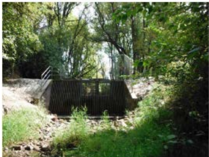
Water Control Structure at Palensky Channel
