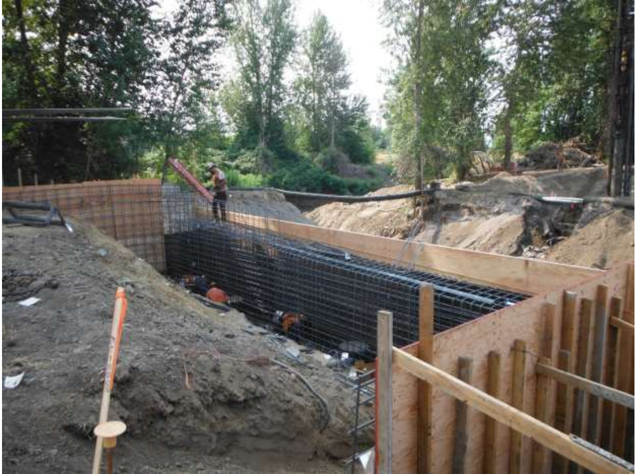
Building the rebar on top of bridge piles and putting up concrete forms
