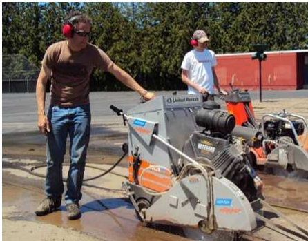
Figure 2 Sawcutters can be used to break pavement into manageable squares, but don’t forget they need electricity and a water source.
